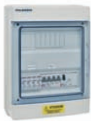
Centralino AC trifase AC three phase panel
